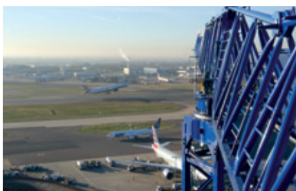
An idea of just how close the crane is to the busy airport
